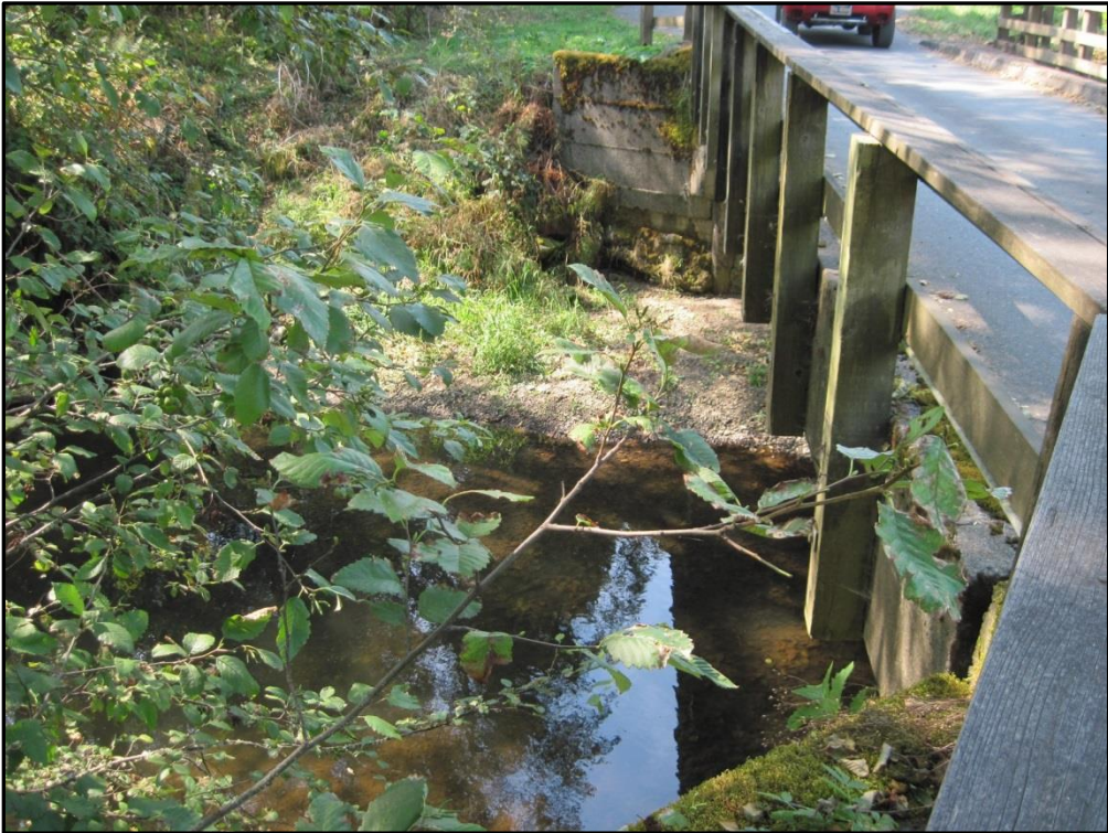
Photo 10: Looking at the upstream end of the bridge from the east side.
