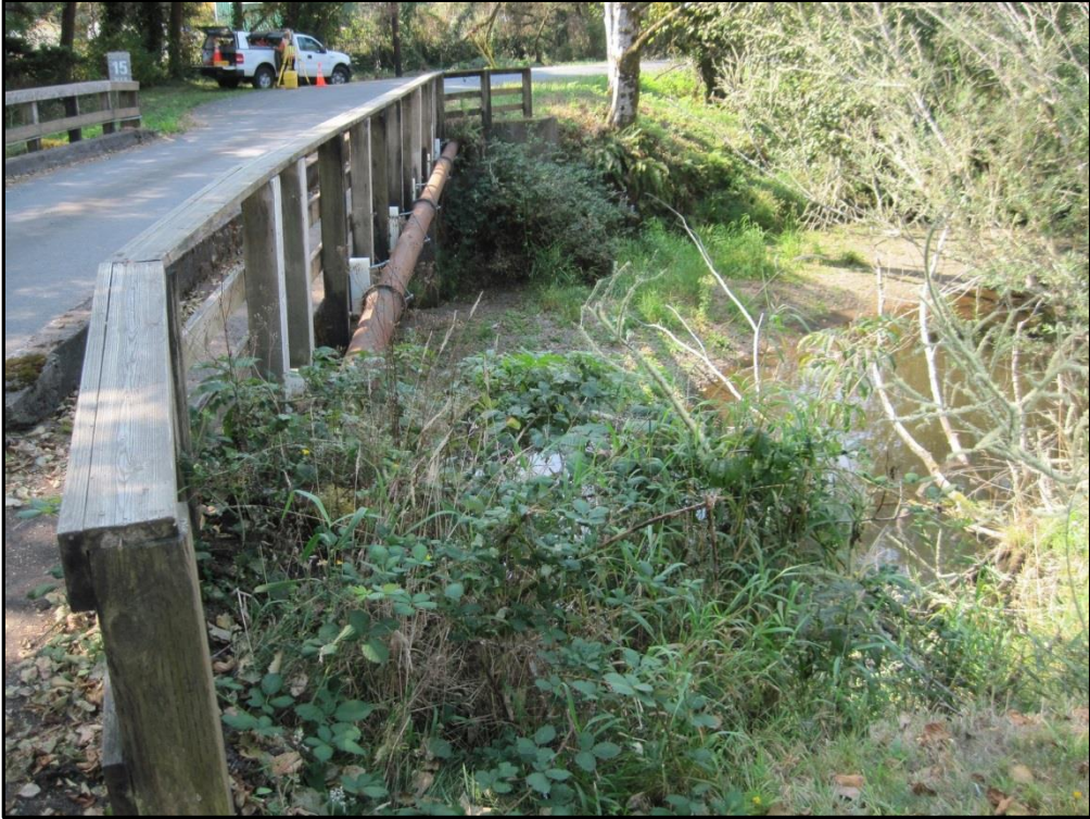
Photo 9: Looking at the downstream end of the bridge from the east side.
